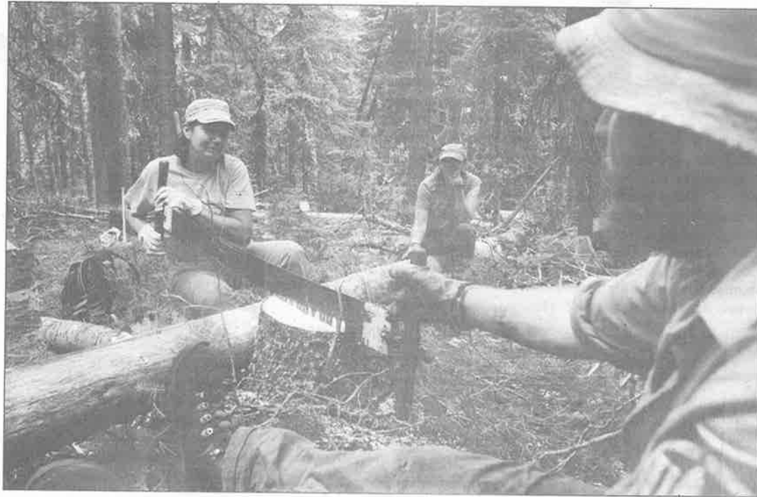
Top: Terry Perkins (center) uses a crosscut saw to low-stump a tree with help from Jeremy Nicholson while Sue Maves waits to rotate in. Middle: U.S. Forest Service Trails and Wilderness Coordinator Kat Barker checks the levelness of logs during bridge construction. Bottom: Back row: David Kallenbach, Kat Barker, Terry Perkins, Walk Hajducki, Sue Maves, Jim Swartz. Front row: KJ Jenkins and Jeremy Nicholson.
